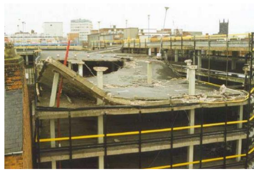
(b) Colapso parcial do edifício Pipers Row Car Park, Wolverhampton (WOOD, 1997)
