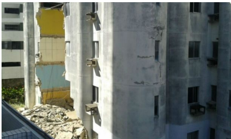
Fig. 1.12. Collapse in Recife [31]
